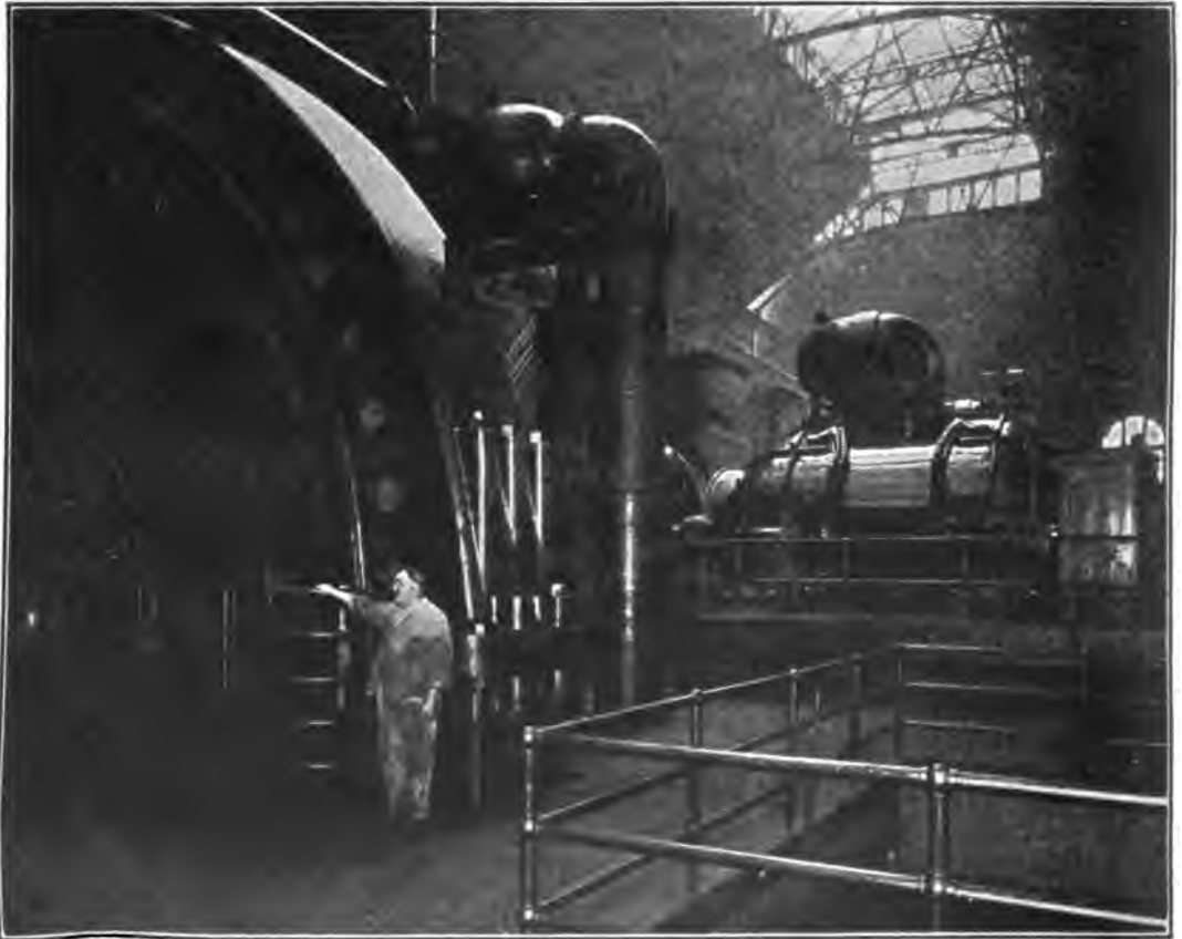
FIG. 2. AT THE LEFT—A SMALL PART OF THE OLD ENGINE; BEYOND, ONE OF THE CYLINDERS OF THE BIG TURBINE
